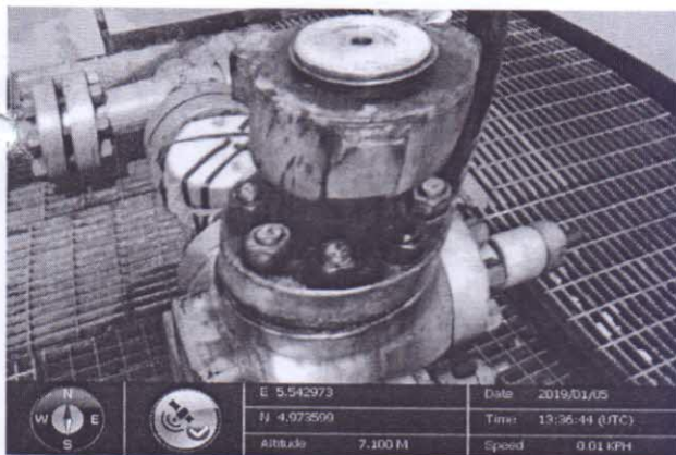
WELL 5T COMPONENT WELLHEAD SHOWN
